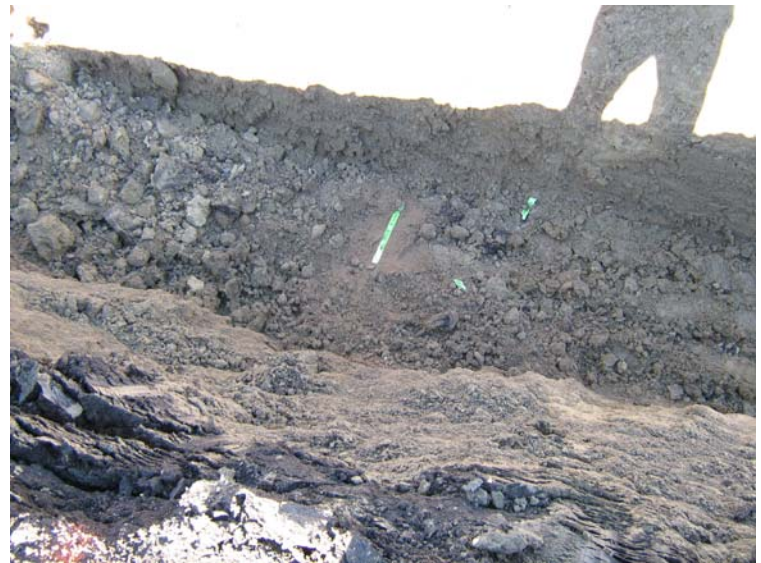
This photo shows the remaining 30" marker visible in the ditch providing a clear indication of the depth of the lines below. No labourers were required in the ditch.
