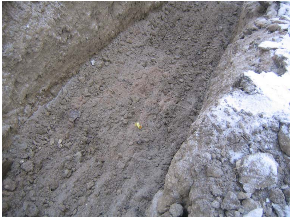
A clean trench over top of the line with the remaining section of Line Alert showing.
