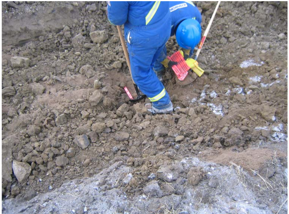
Workers hand exposing the line digging down the sides of the Line Alert panel providing guidance to the worker. Note the yellow sections (13"-24") and red sections (1"-12") providing clear depth indication from the buried line.
