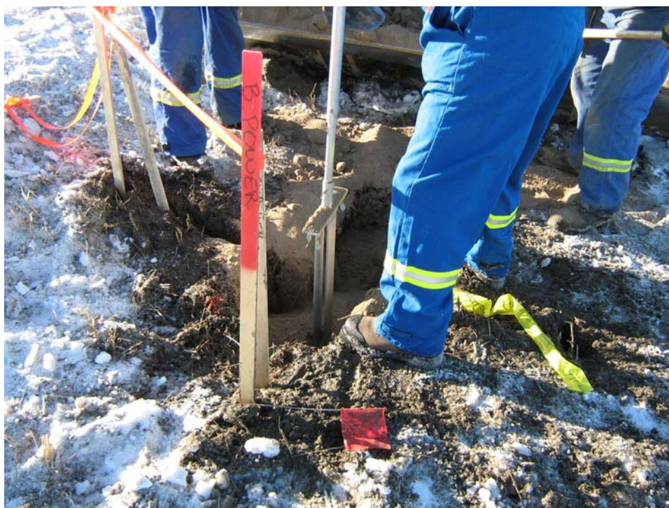
The Line Alert panel has been backfilled to the top and the installation tool is being removed. Note the yellow "Line Alert Installed" caution tape between the feet of the worker. The caution tape is attached to the panel and runs to the surface providing an installation marker.
