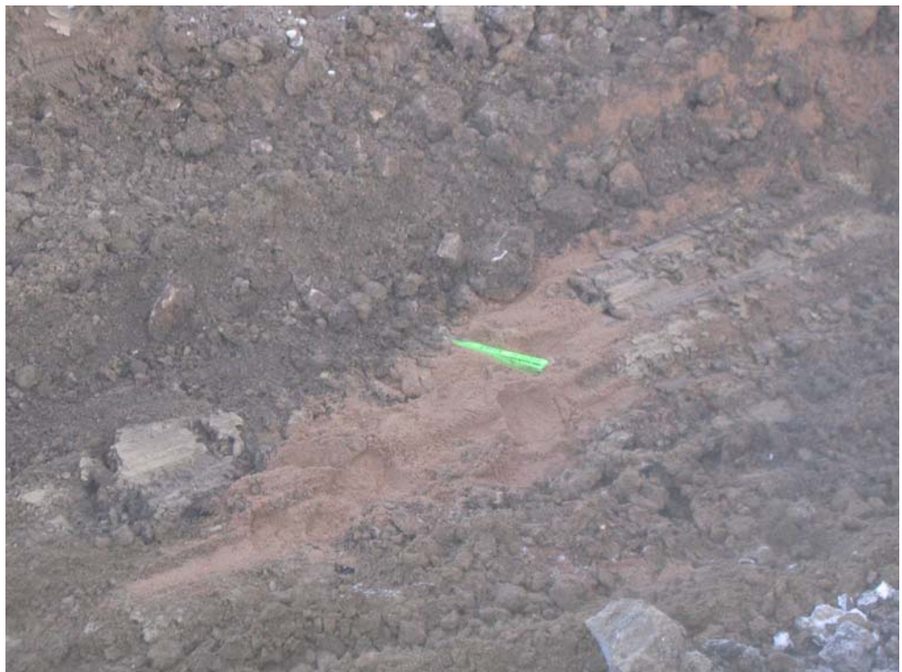
A clear image of the green section of the Line Alert panel showing in the ditch following a bucket pass. Note how even in the frost conditions with large chunks of soil, the panel indicators are still highly visible.
