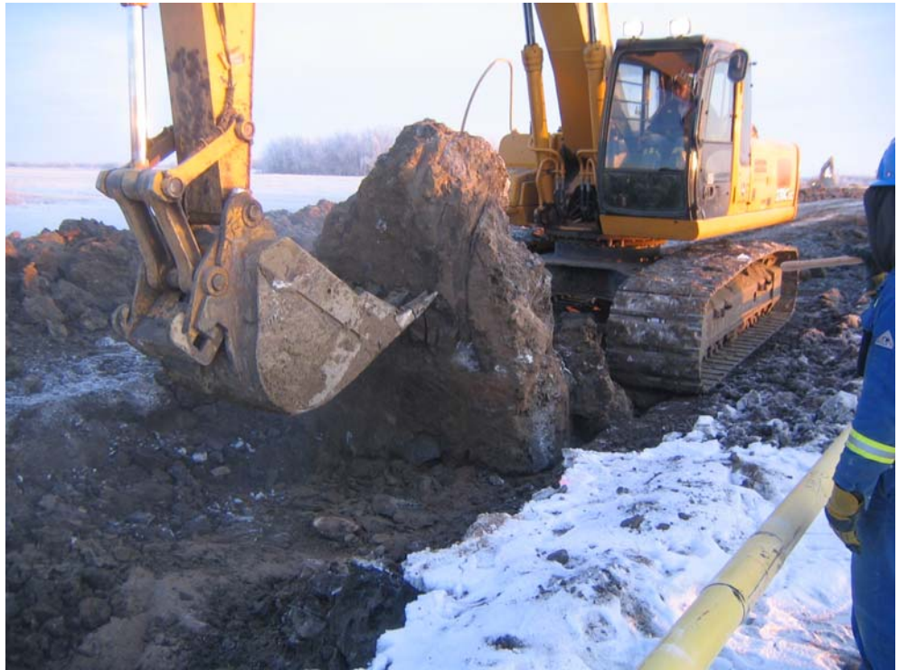
This photo shows the extreme soil conditions caused by frost during this excavation work.
