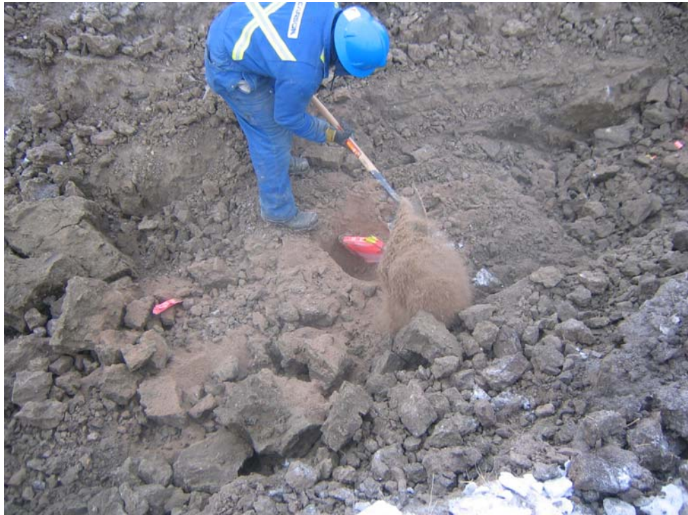
Using the Line Alert panel as a guide to stay away from the line while hand exposing the line.
