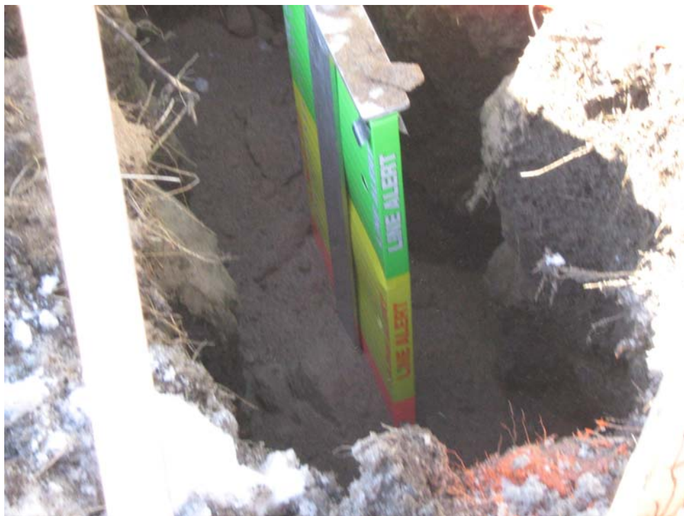
The Line Alert panel being held in place on the line by the installation tool as the hole is backfilled with sand.
