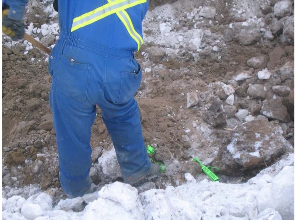
Worker clearing frost chunks to confirm the depth on the Line Alert sections after the bucket first encountered the panel.
